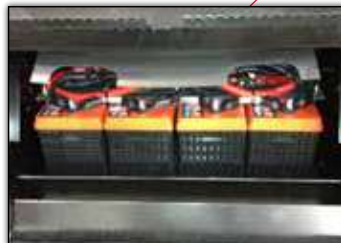
Four Group 31 batteries, electrically isolated from the truck, power the system.
